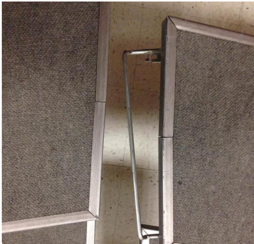
Figure 1: Madison Middle School's current risers do not join together properly.
